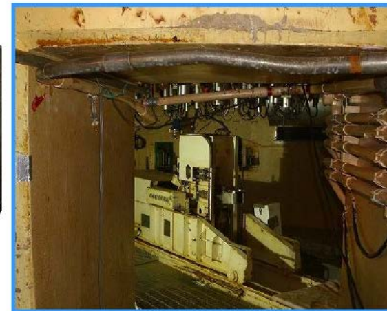
(Reference information) Pedestal opening of Unit-5
