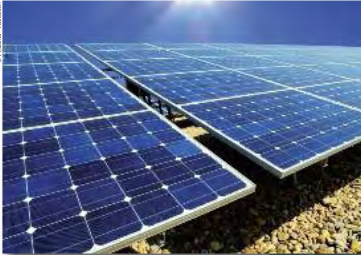
Photovoltaic panels have been installed in the stadiums and World Cup cities.
